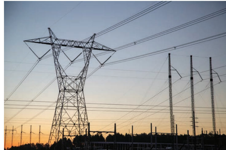
Our electric grid gathers and distributes power from many sources, including power plants that convert fossil fuels like coal, natural gas and oil into electricity; nuclear power plants; and renewable energy sources, such as wind turbines, solar farms, hydroelectric dams and even landfills.
