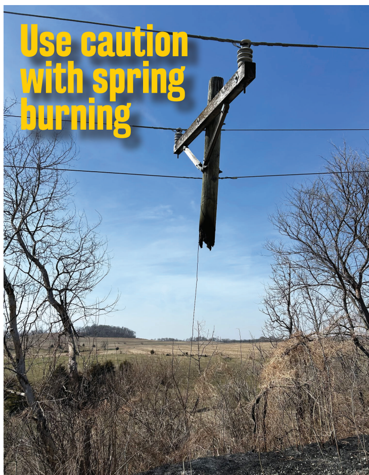
This is a photo of a MiEnergy pole taken the week of March 23. It is a good reminder to use caution when burning near power lines. Beyond power poles, there can be cabinets, transformers for underground service and guy wires hidden in the tall grass or other overgrown vegetation. If these burns are not managed safely, they can cause property damage, power outages, injury, and even death. Burning a power pole or other electrical equipment could cause a widespread power outage and be costly for the individual responsible for the fire.
