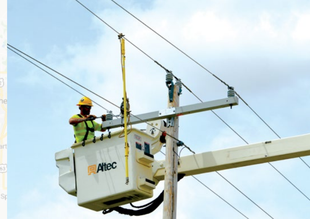
Clint Lickteig working on a project that added three-phase electric lines to transport power from Madison Solar to the Madison Substation.
